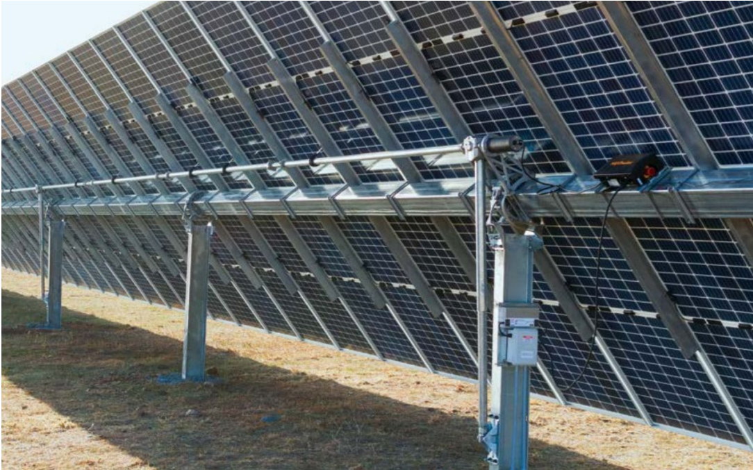
STABLE AT FLAT STOW Nextracker's 2P NX Gemini tracker—shown here at the National Renewable Energy Laboratory's (NREL) Flat Irons Campus for wind testing in Boulder, Colorado, U.S.A.—incorporates self-locking linear actuators at each foundation to ensure stability against dynamic wind effects.
